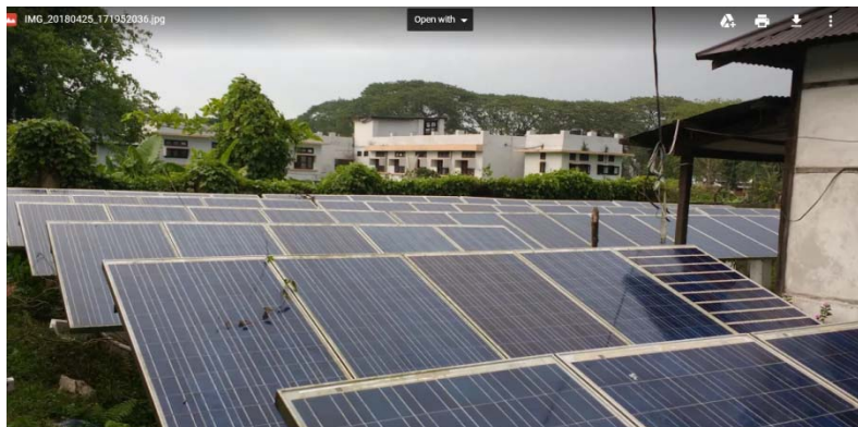
Figure 9: Solar panels installed at the GUIST campus that generate ~40KW of power
